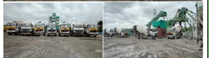
Ready-Mix Concrete Plant at IDA Bolaram
